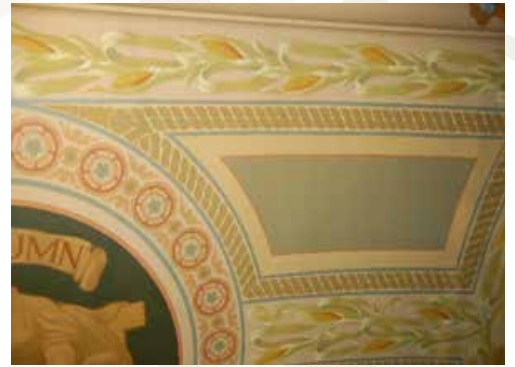
Minnesota State Capitol. Photos courtesy of John Canning & Co., Decorative Painting and Restoration Contractor
